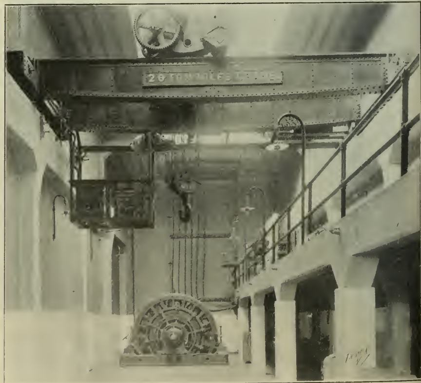
FIG. 16. INTERIOR OF SUBSTATION
